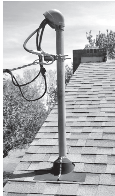
Electrical Mast Roof Flashing
