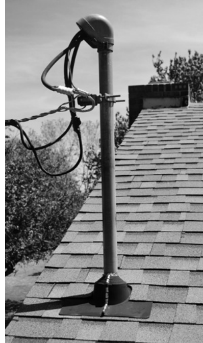
Electrical Mast Roof Flashing
